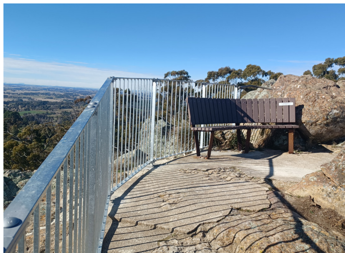
Fence replacement project at Pinnacle Lookout, Orange funded by Crown Reserve Improvement Fund 2022–23
