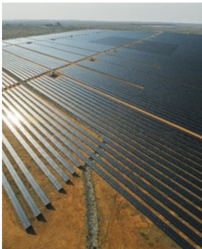
Broken Hill Solar Farm
