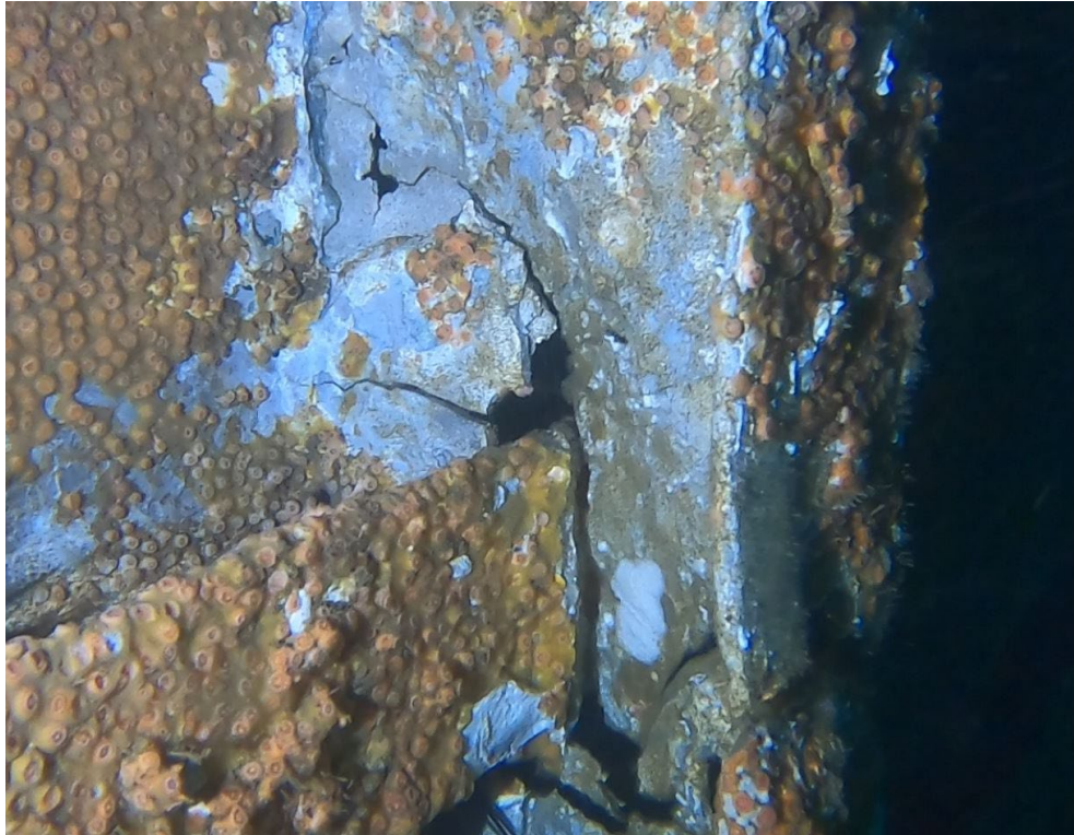
Figure 16: This is a typical aluminum frame and stringer on the exterior wall of 01 deck. The walls are breaking down due to cracking and corrosion and then the panels break off the superstructure.
