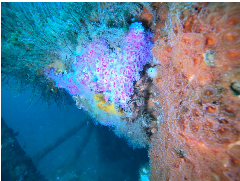
Figure 21: The mast is in sound condition and is heavily encrusted with colourful marine life.
