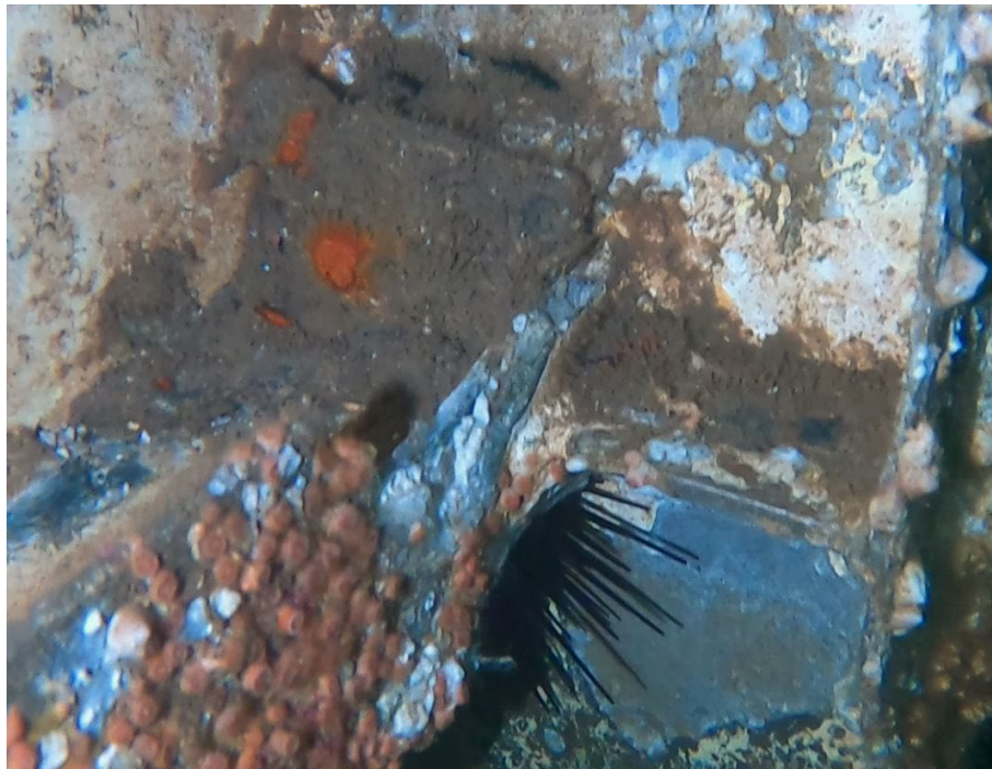
Figure 17: An example of the corrosion in the heat affected zones of the stringer connections to the frames.
