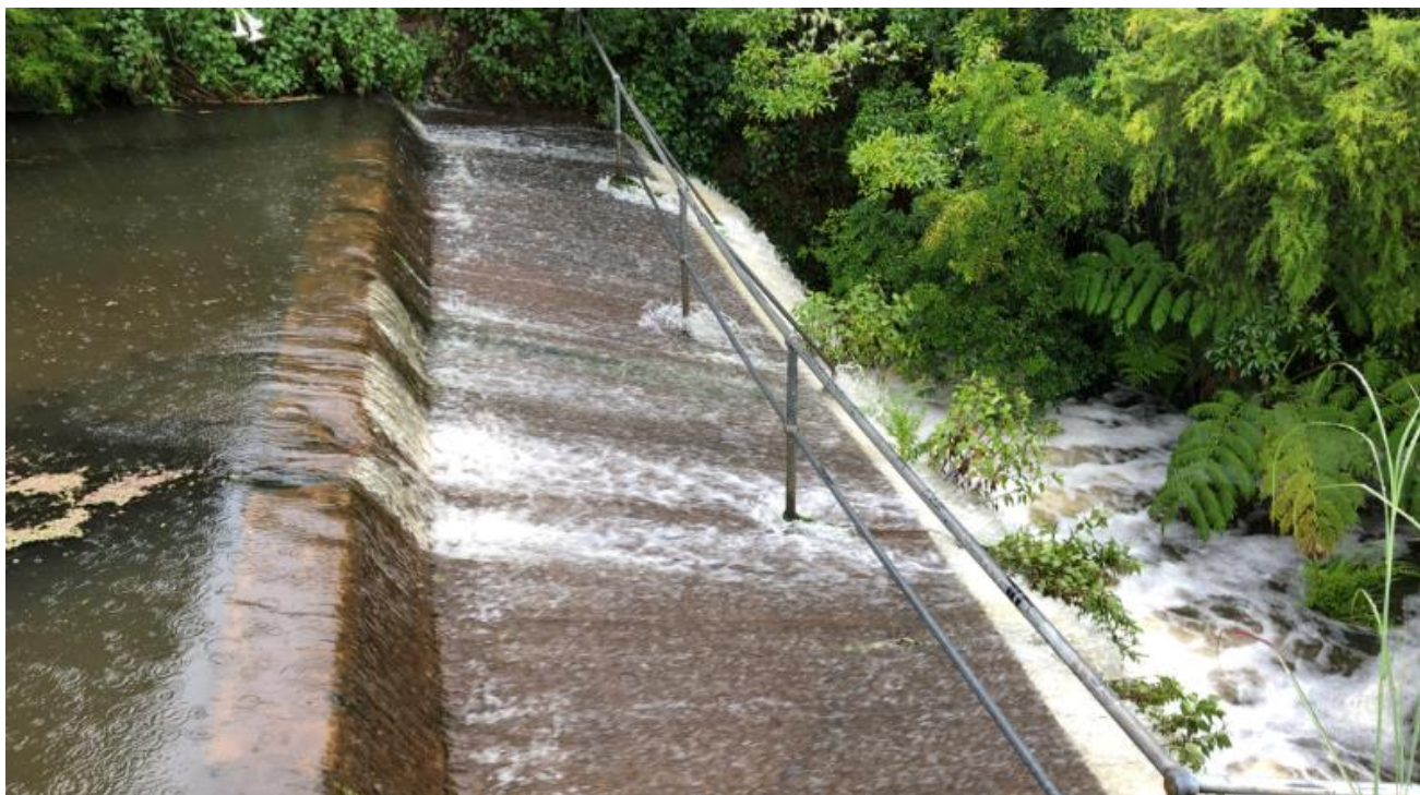
Figure 4.6 Overtopping of the spillway during a rain event
