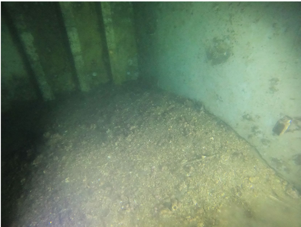
Figure 37: The silt build-up in the enclosed compartment against the starboard wall. This is the location that the opening in figure 10 was made
