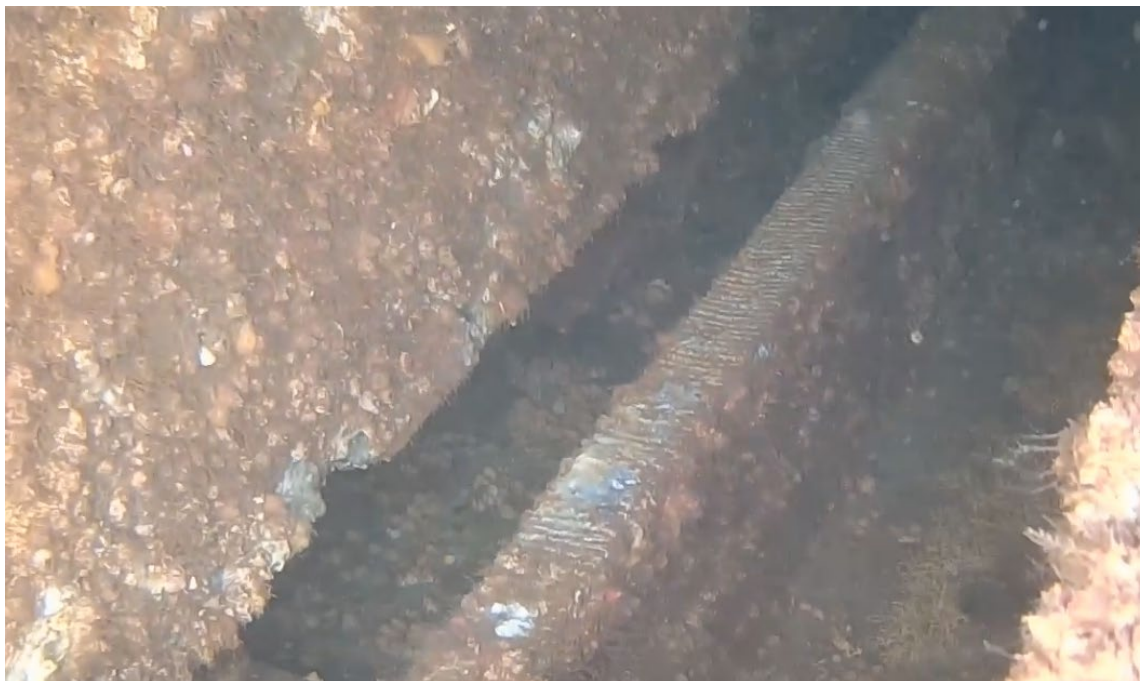
Figure 7: The separated hanger wall to the left and the 100mm high steel stub on the main deck that it was welded to. The aluminum superstructure is breaking off along this seam in many places on the main deck.
