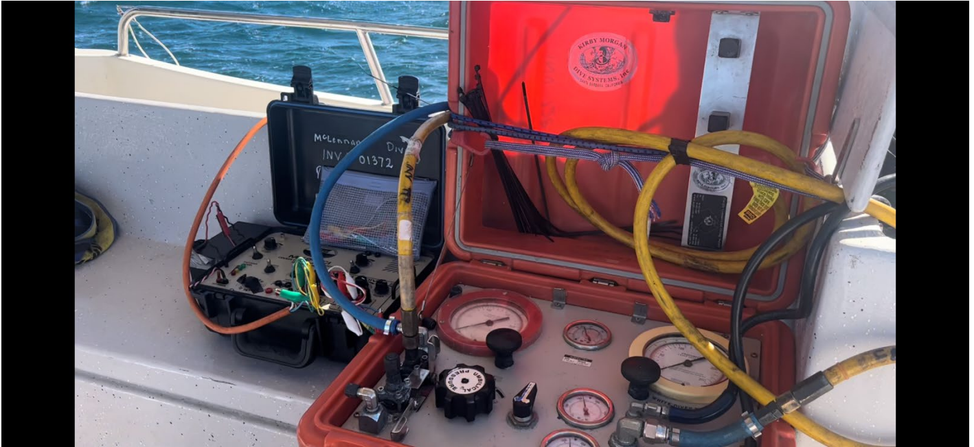
Figure 38: Diver gas control panel and communications box
