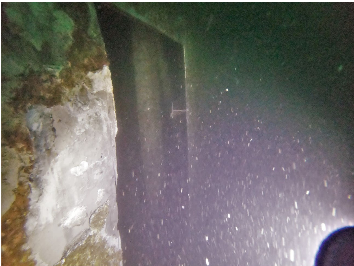
Figure 11: The opening cut into the outer starboard wall shown above measuring 1700mm by 800mm
