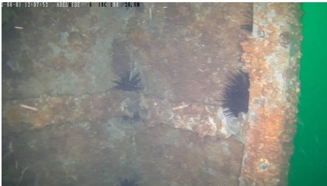
Figure 5: The aft supporting column of the starboard hanger looking from inboard. The column shows no sign of deterioration. The similar column on the port side showed cracking and crumpling in the weeks before the hanger collapsed.
