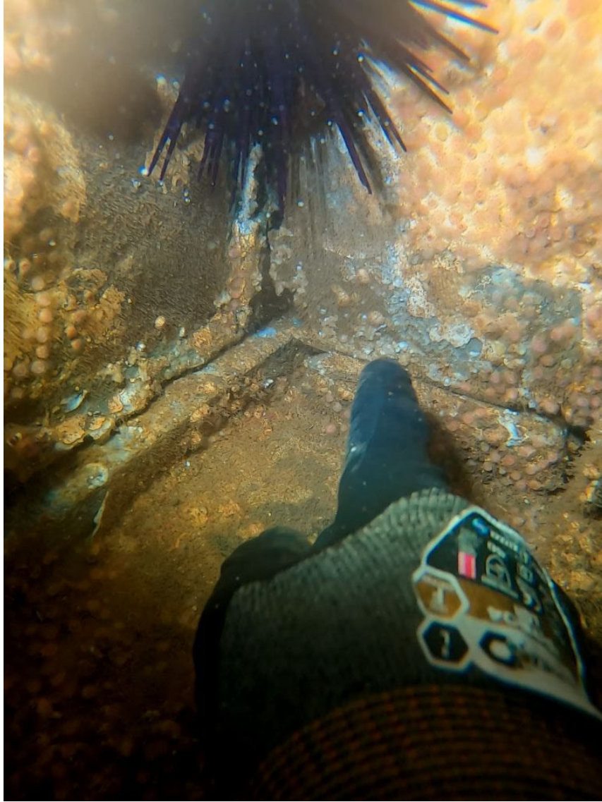
Figure 2: The divers hand pointing to the separation of the hanger companionway wall from the main deck. It is not currently presenting any dangers due to objects nearby holding it in position
