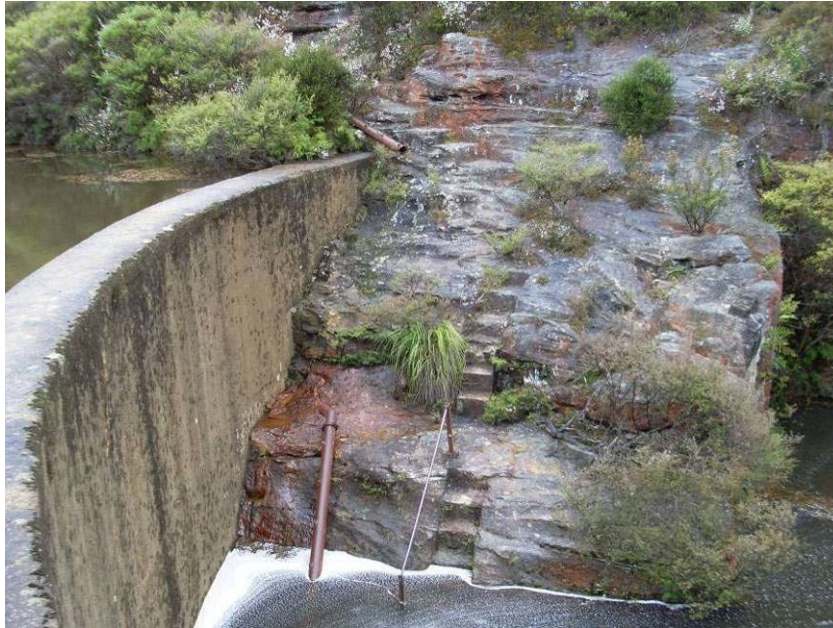
Plate 10: The upper dam wall and associated infrastructures requires a cultural heritage assessment
