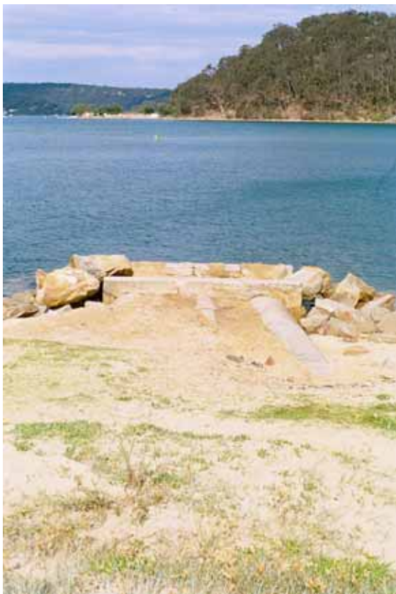
Figure 34 - Stormwater outlet near Lemon Grove Reserve entrance
