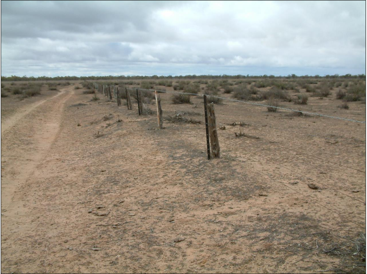
PLATE 18. Mapping Area B- The fence eastward of that shown in Plate 17 needs replacement (15/08/2008).
