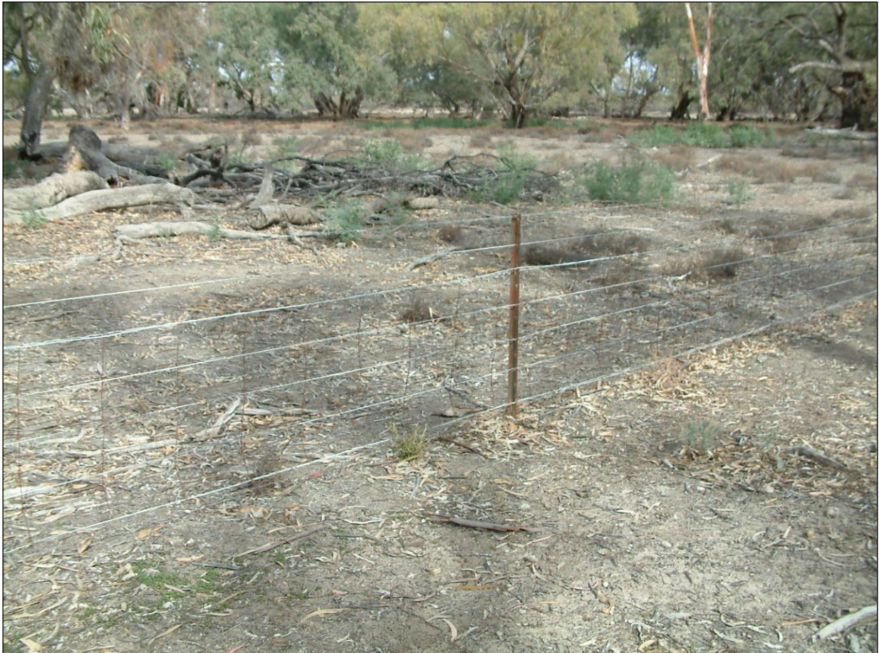
PLATE 11. A section of the boundary between the Menindee Common and Appin Station, renewed entirely by Appin Station (15/08/2008)
