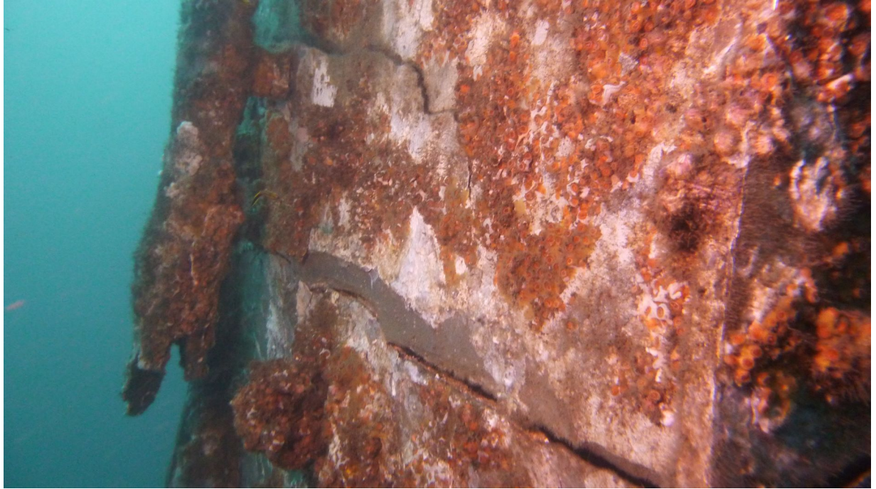
Figure 3: The break in one face of the port hanger column
