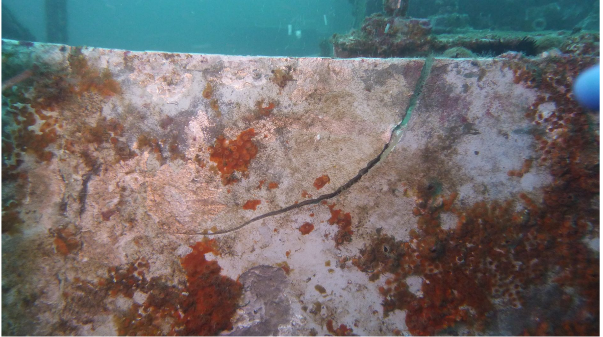
Figure 7: This is the break through the aft face of the hanger wall above the hanger door.
