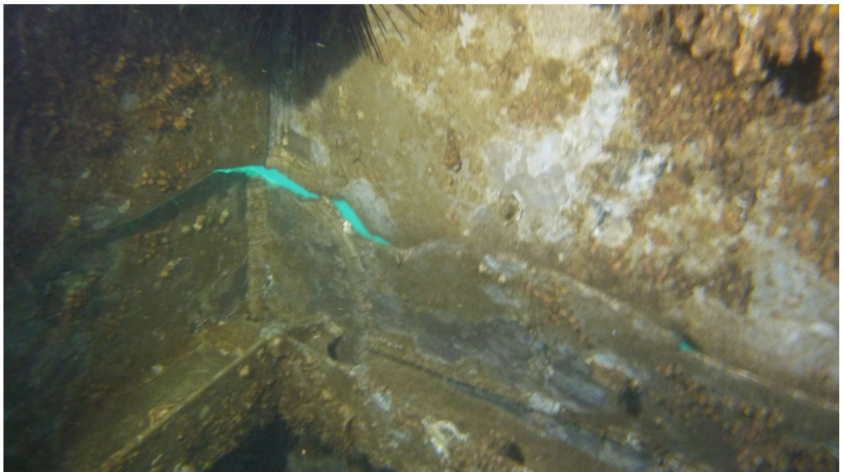
Figure 6: This view shows the cracks through the port side column from the inside
