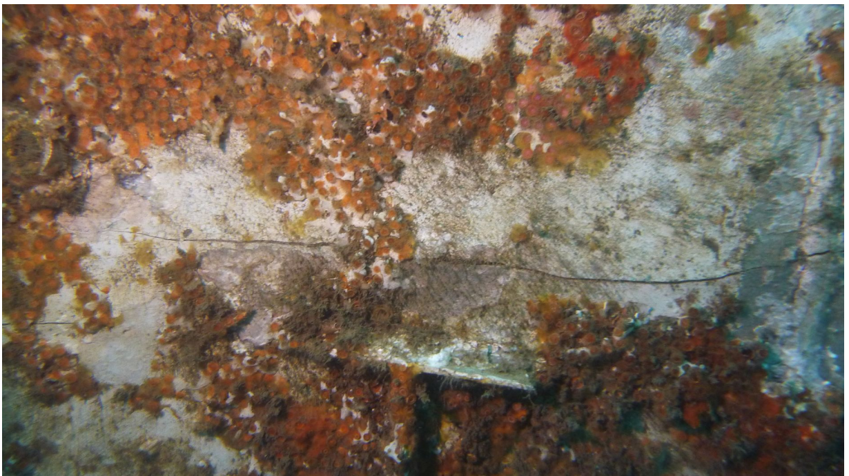
Figure 8: This is the same crack shown above but shows it travelling along the aft wall
