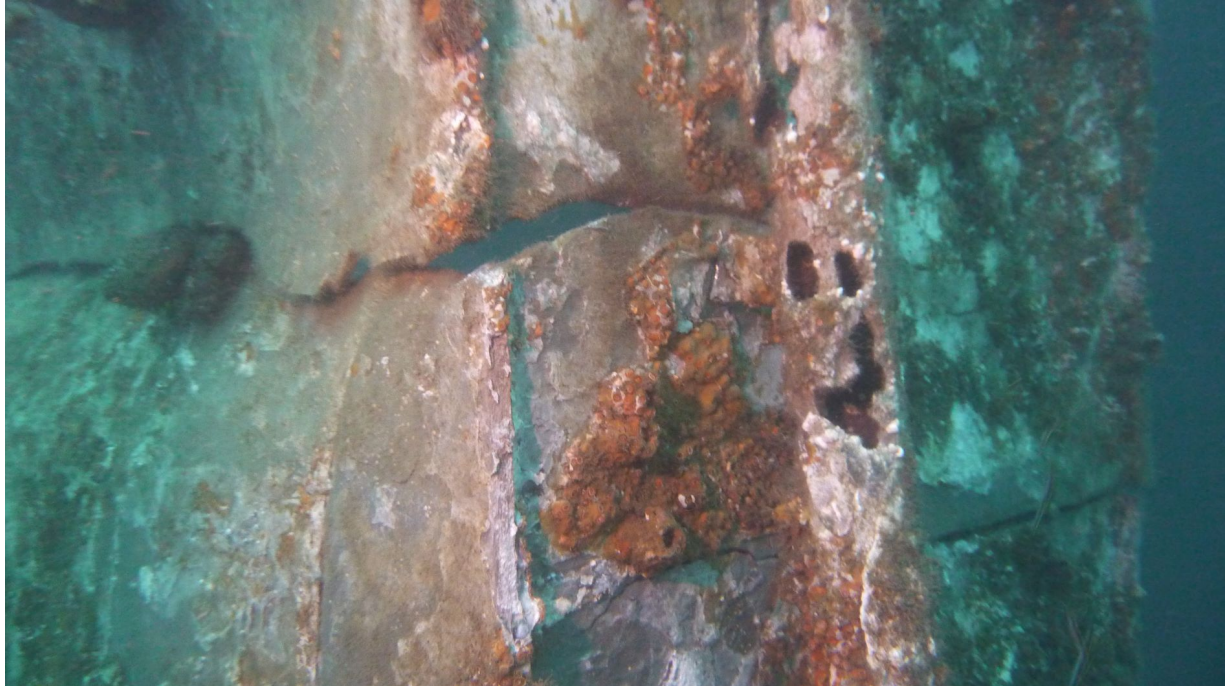
Figure 5: A view of the corner of the port side column. This shows the same cracks as in Figures 1 and 2
