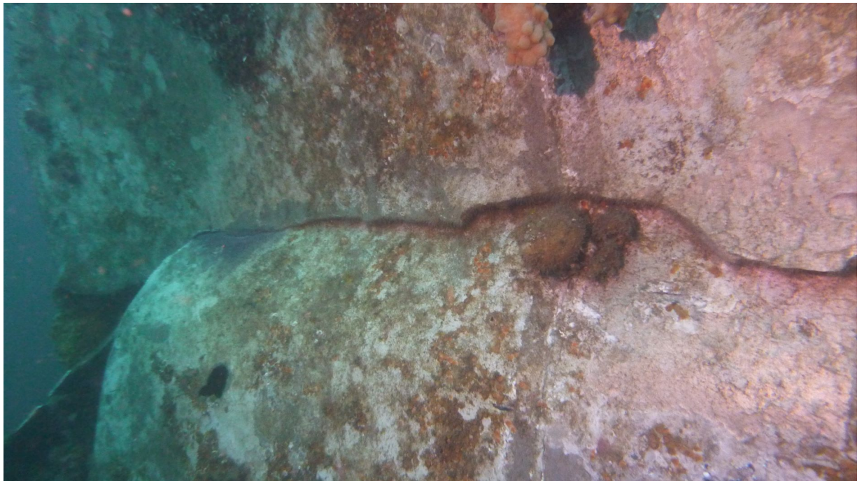
Figure 4: The break in the outboard face of the hanger column. Not the compression of the column
