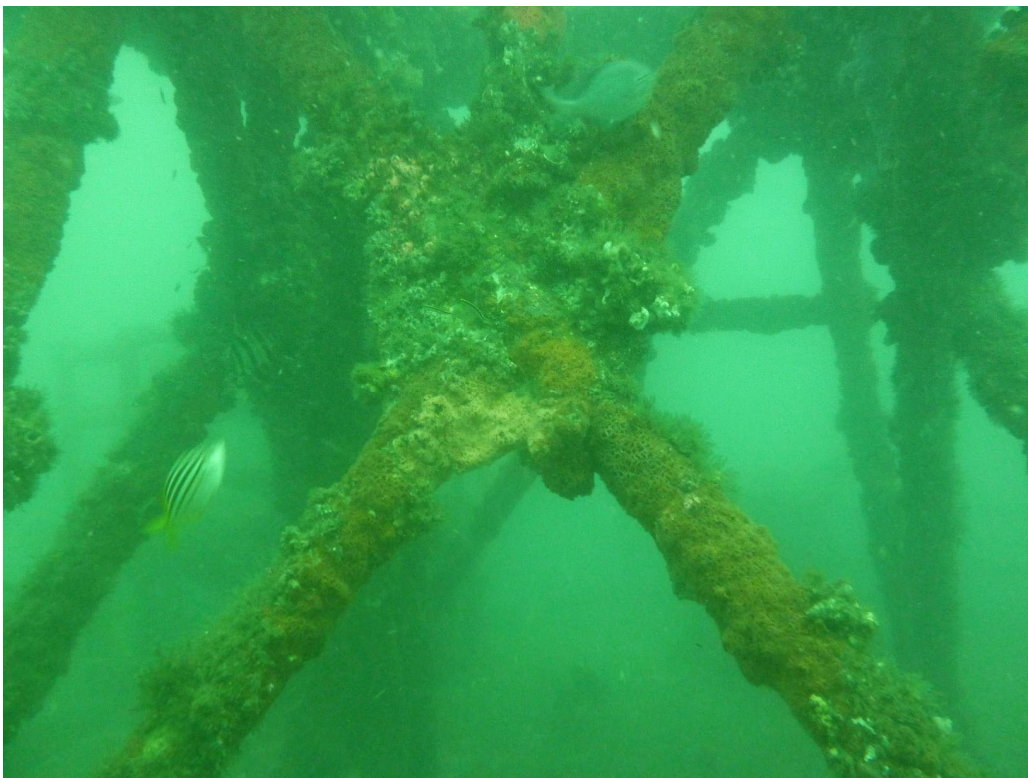
Figure 14: A close-up of the strut of the main mast. It is fully encrusted with marine growth and no sign of corrosion or cracking.
