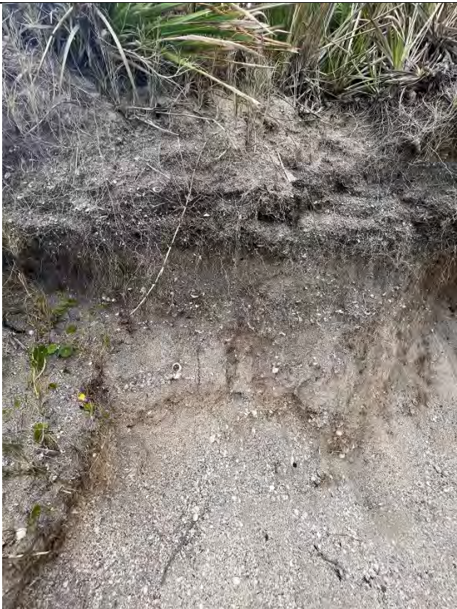
Character of the potential Aboriginal shell midden and impacts of erosion to be remediated.
