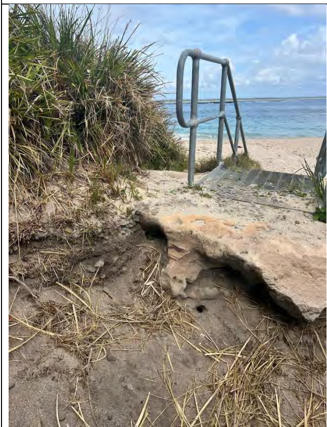
Character of the steel staircase and eroded sandstone. Photograph taken looking in a westerly direction.
