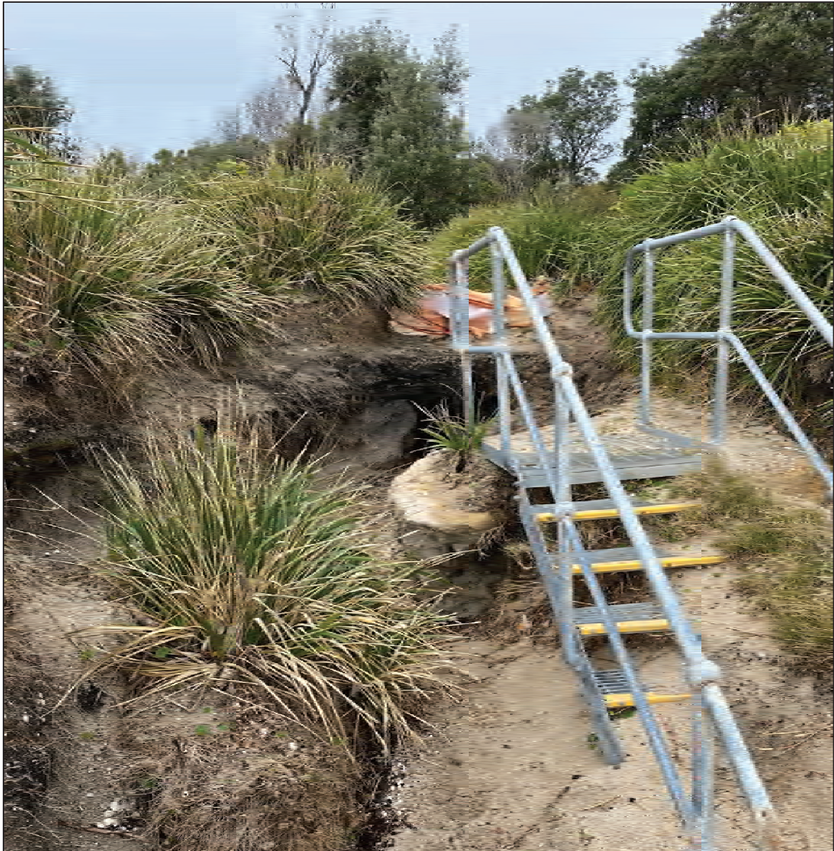
Figure 2: Base of stairs leading onto Wilsons Beach showing erosion of potential shell midden (Source: NSW Crown Lands)
