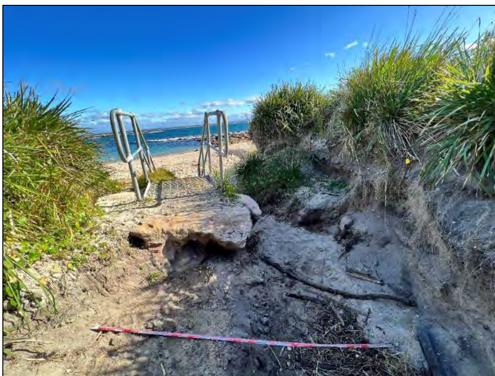
Plate 8: View across staircase towards beach, showing level of erosion present.
